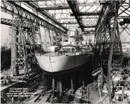
USS Alabama being constructed on Norfolk Naval Shipyard's Building Ways during World War II. Photo by Earl Parsons, head photographer. NNSY Archives.
